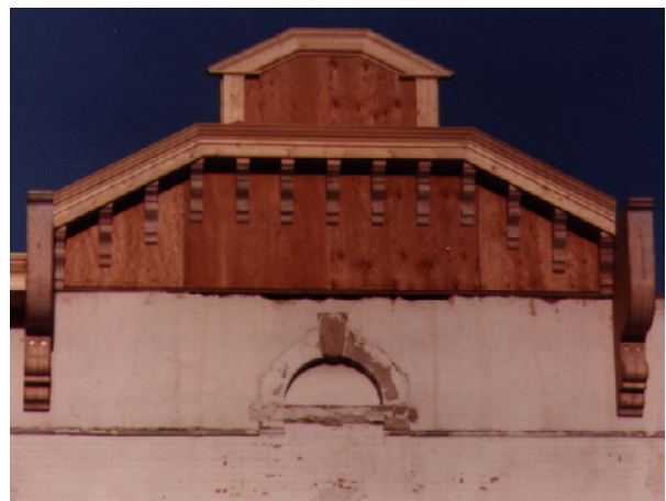
The pediment of the Reed & Dauthe building during reconstruction, in compliance with the Old Town design guidelines.
