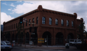
The parking facility and new downtown civic plaza in Flagstaff, Arizona, was under construction in the summer of 1998.
